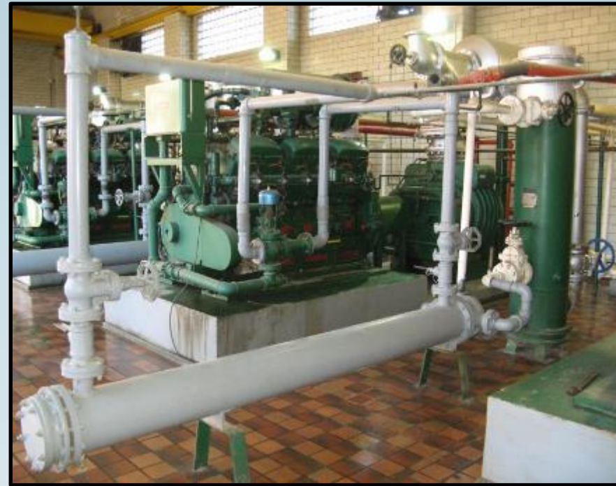
Biogas Fueled CHP Systems
