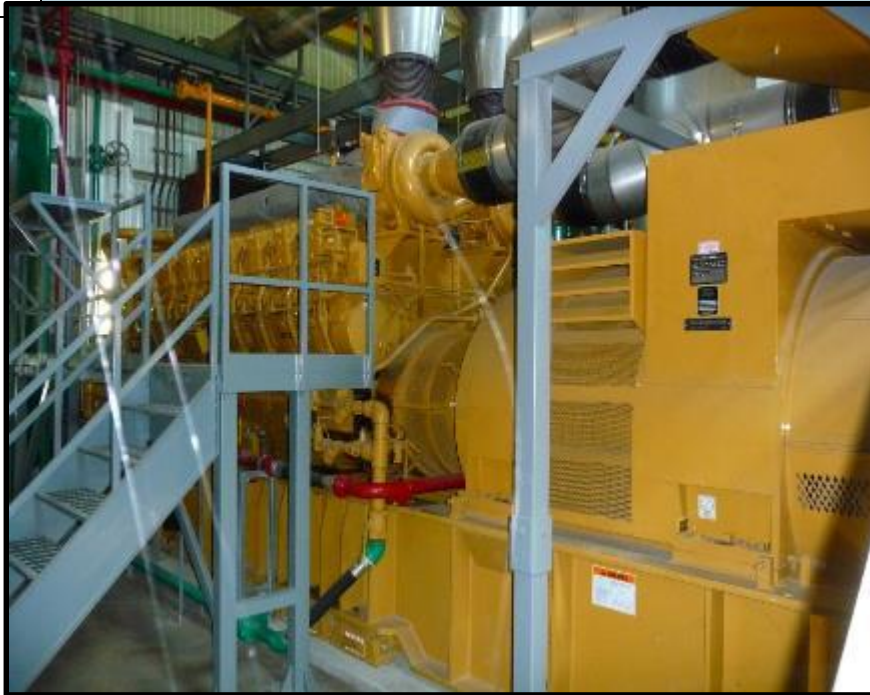
Standby Power Generator Systems
