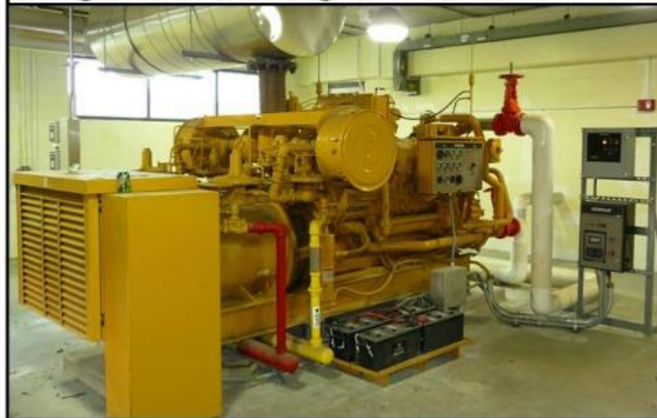
Biogas Fueled Engine-Generator
