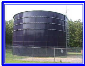
Vesper View Water Storage Tank
